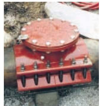
Mechanical line stop fitting with blind flange.
