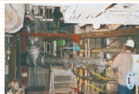
8" (200mm) HTP line stop on steam condensate line.
