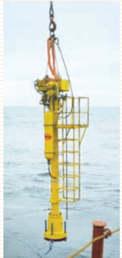
914XL hot tap machine is lowered into North Sea for 16" hot tap.
